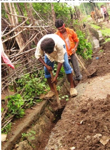
Cleaning area next to hand pump at Dewada, Tadoba
