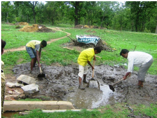
Pit being dug to create water body next to hand pump at Fulzari, Pench (Mah)
